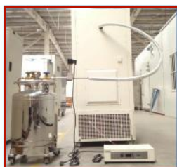
LN 2 /CO 2 backup system
